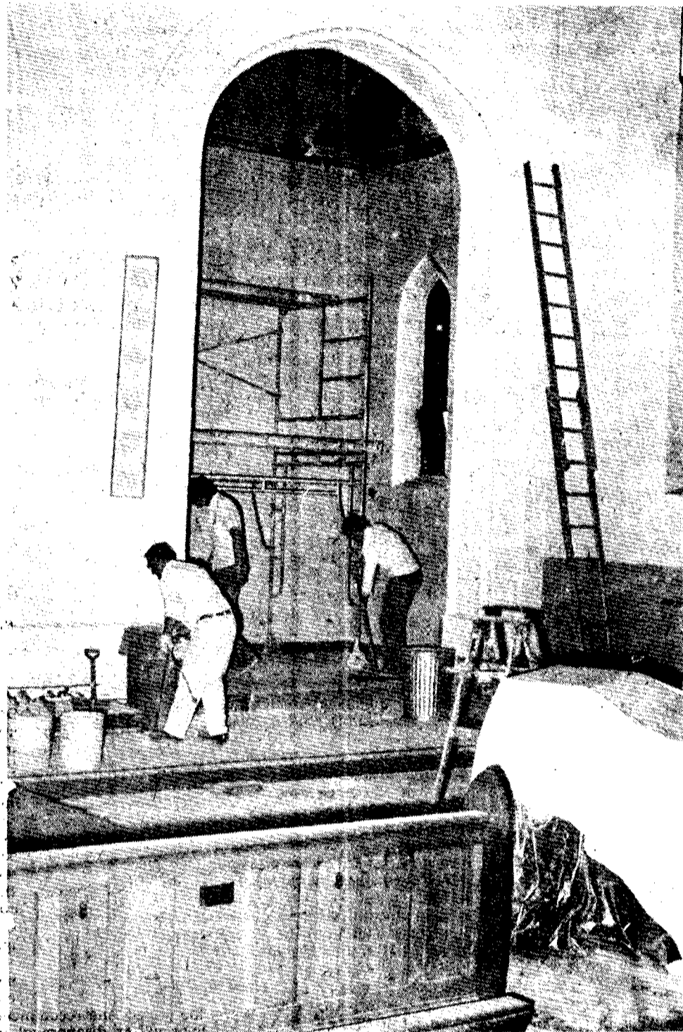
RENOVATION WORK in the sanctuary of St. Agatha's Catholic Church in Gagetown got underway Wednesday, April 4. It is to be done in time for the church's 100th anniversary celebration June 4.
