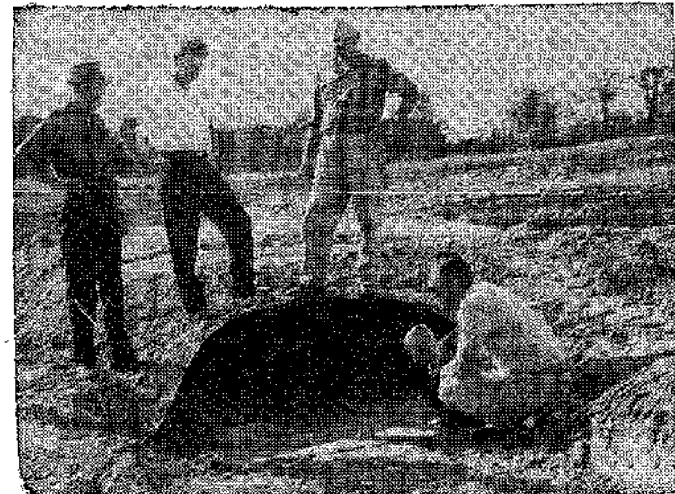
ONE OF MANY —When the huge project is completed, more than 200 erosion control structures will be installed. A tube of this type will collect water from over 150 acres and drop it safely into the river without eroding the river bank and filling the channel. Shown here is the entrance.
