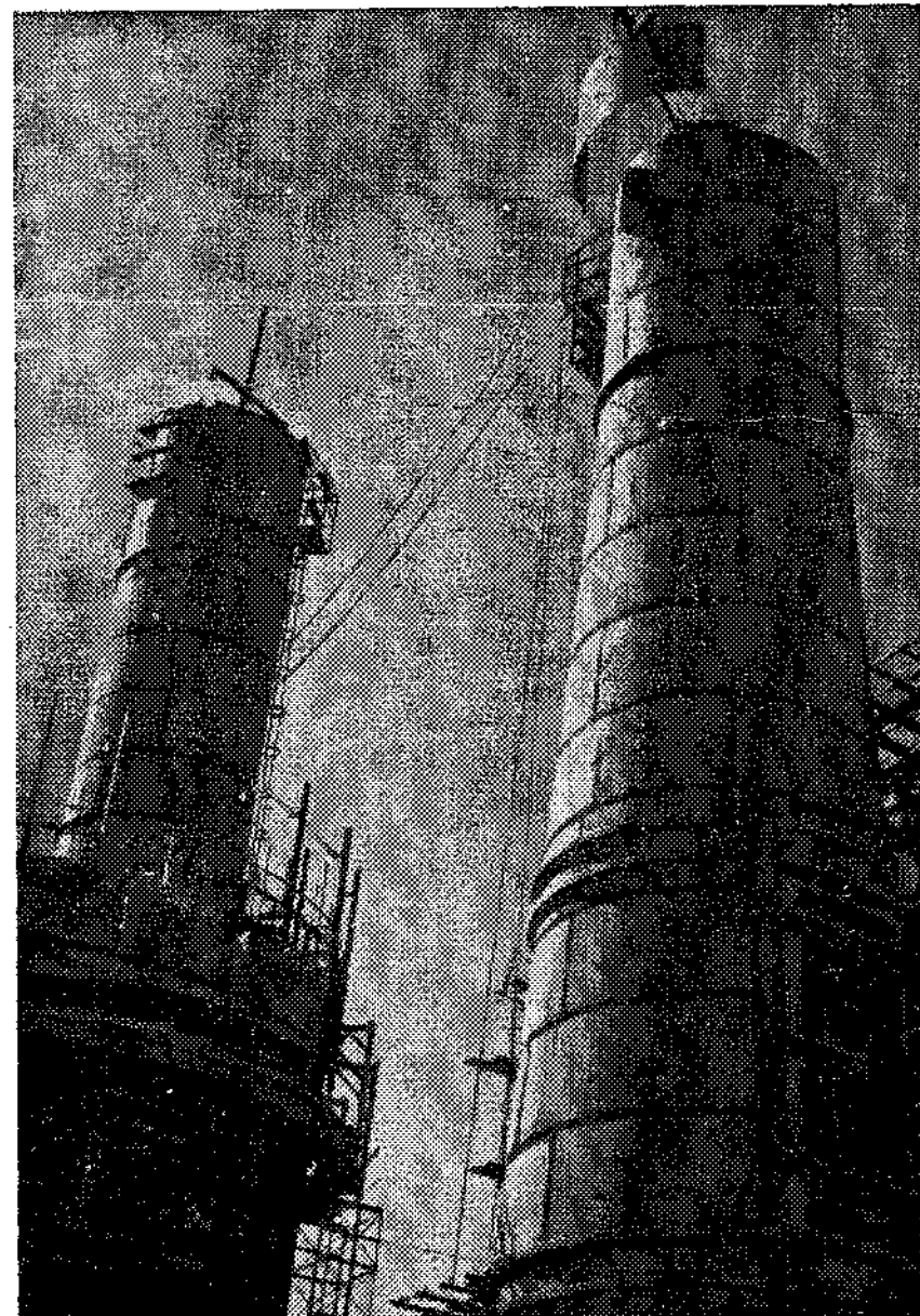
GOING UP! Two of the four stacks, which will finally reach a height of 250 feet, are pictured here. One generating unit is nearing completion and will be in operation by August 1953.
