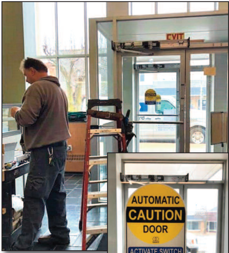
THE LATEST upgrades at the Cass City Municipal Building include installation of American with Disabilities Act (ADA)-compliant doors with an automatic door opening system at the front entrance.
