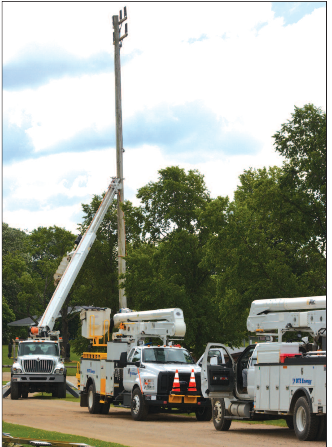
DTE, shown here installing light poles, has been instrumental in work done on Cass City recreational park fields.
