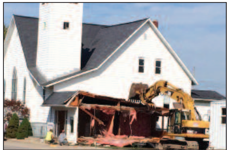
BOOMS Construction demolished the entrance to the Owendale United Methodist Church in preparation for renovations and construction to add an elevator, restrooms and a new office area.
