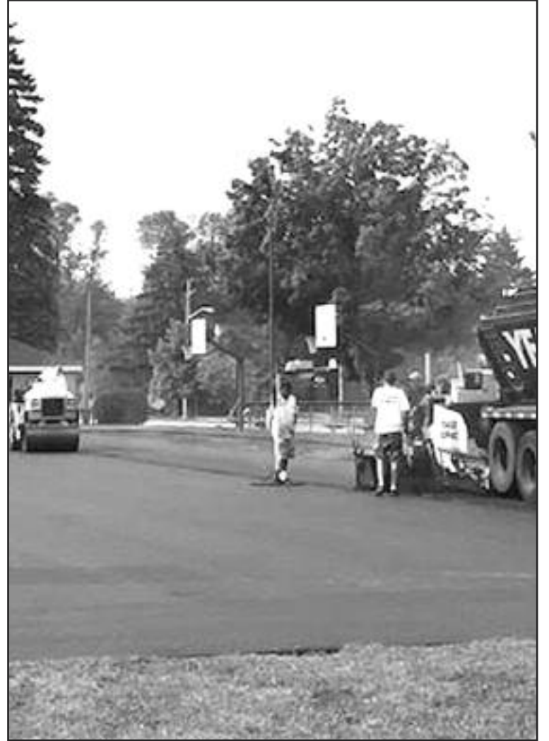
A LONG AWAITED project was set in motion last week as crew members for Yeager Asphalt resurfaced the basketball courts in Cass City Recreational Park.
