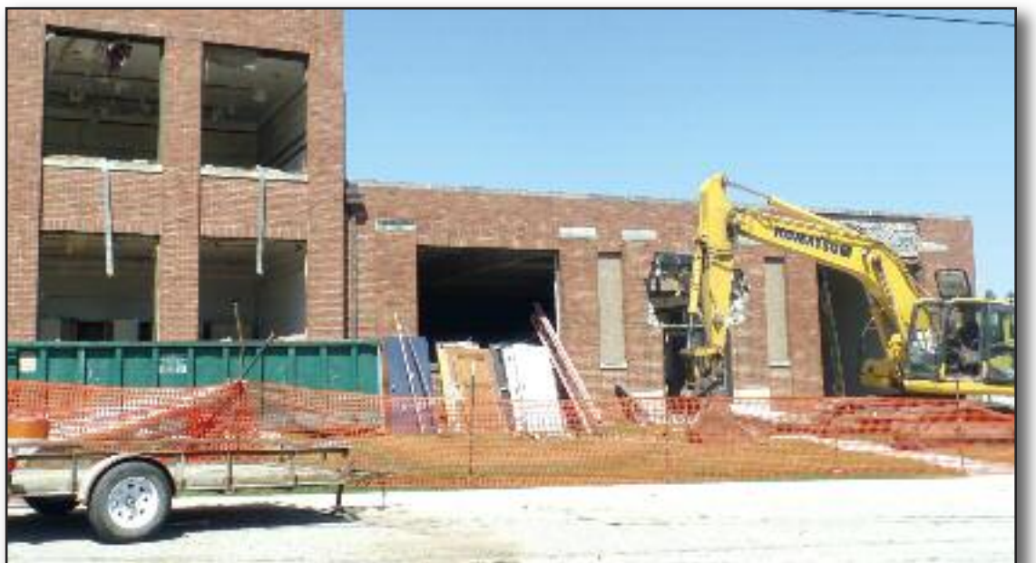
LJ CONSTRUCTION workers have started demolishing the oldest part of Kingston Elementary School. The first portions to go were the interior and exterior doors and windows.
