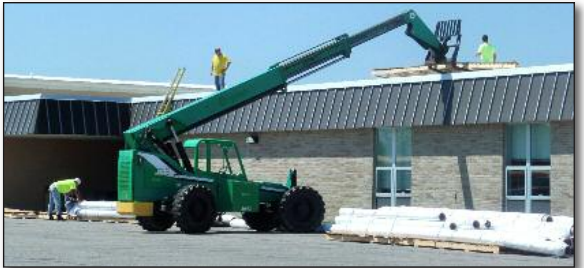
A WORK CREW from Zimmer Roofing has been busy with roof work at Kingston School District’s Junior-Senior High School as part of the district’s $4.8 million renovation, demolition and upgrade project.
