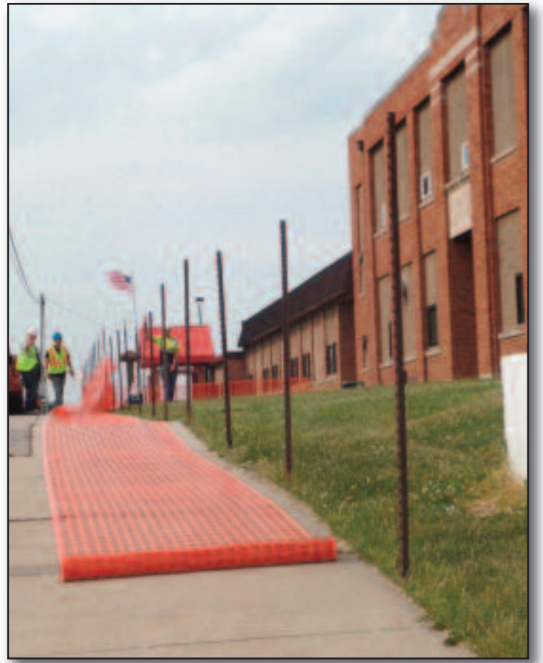
WORKERS FROM LJ Construction were recently in Kingston to install a fence in preparation for when a portion of Kingston Elementary School will be razed.
